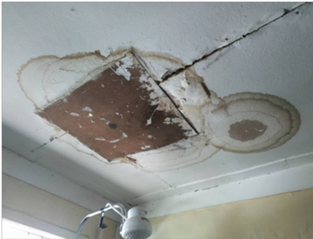
Il. 10. Damaged part of the building | former Polish Club (the timber – framed part)
